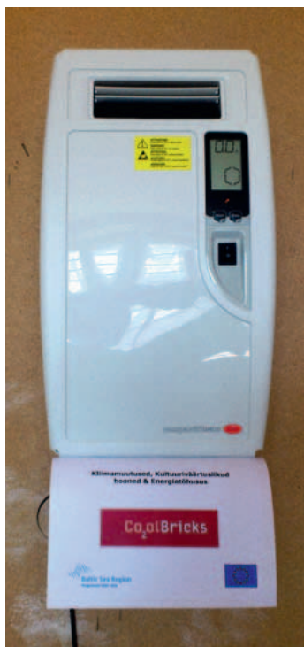
Humidifier in school building, Kohtla-Järve, Estonia
